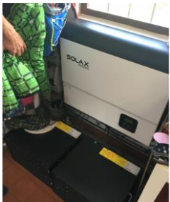
Figure 11: Battery storage unit
